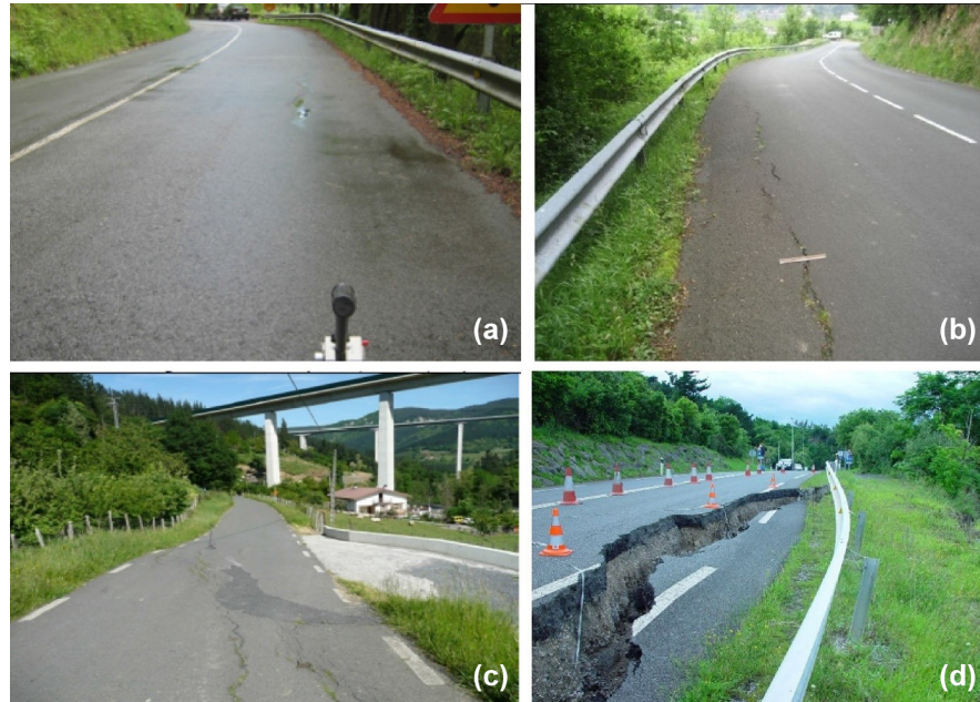
Figure 1.2: Road damage severity classification: (a) no/slight damage, (b) moderate damage, (c) severe damage, and (d) partial/total destruction [6]
