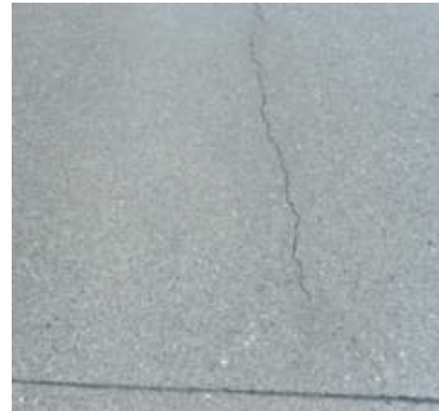
Fine crack in asphalt
