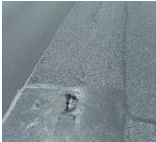
Pothole (7cm depth)
