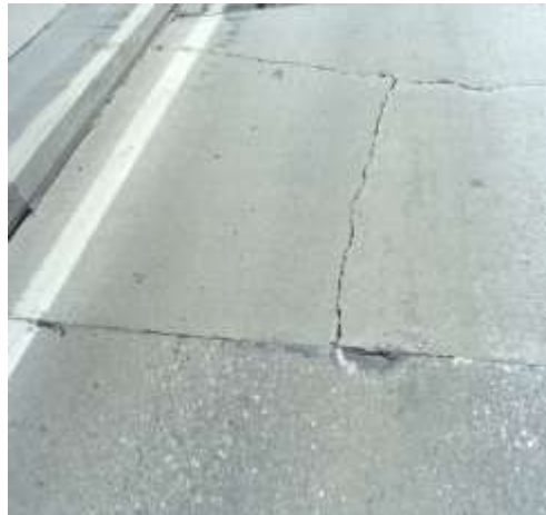
Concrete cracks and detachment
